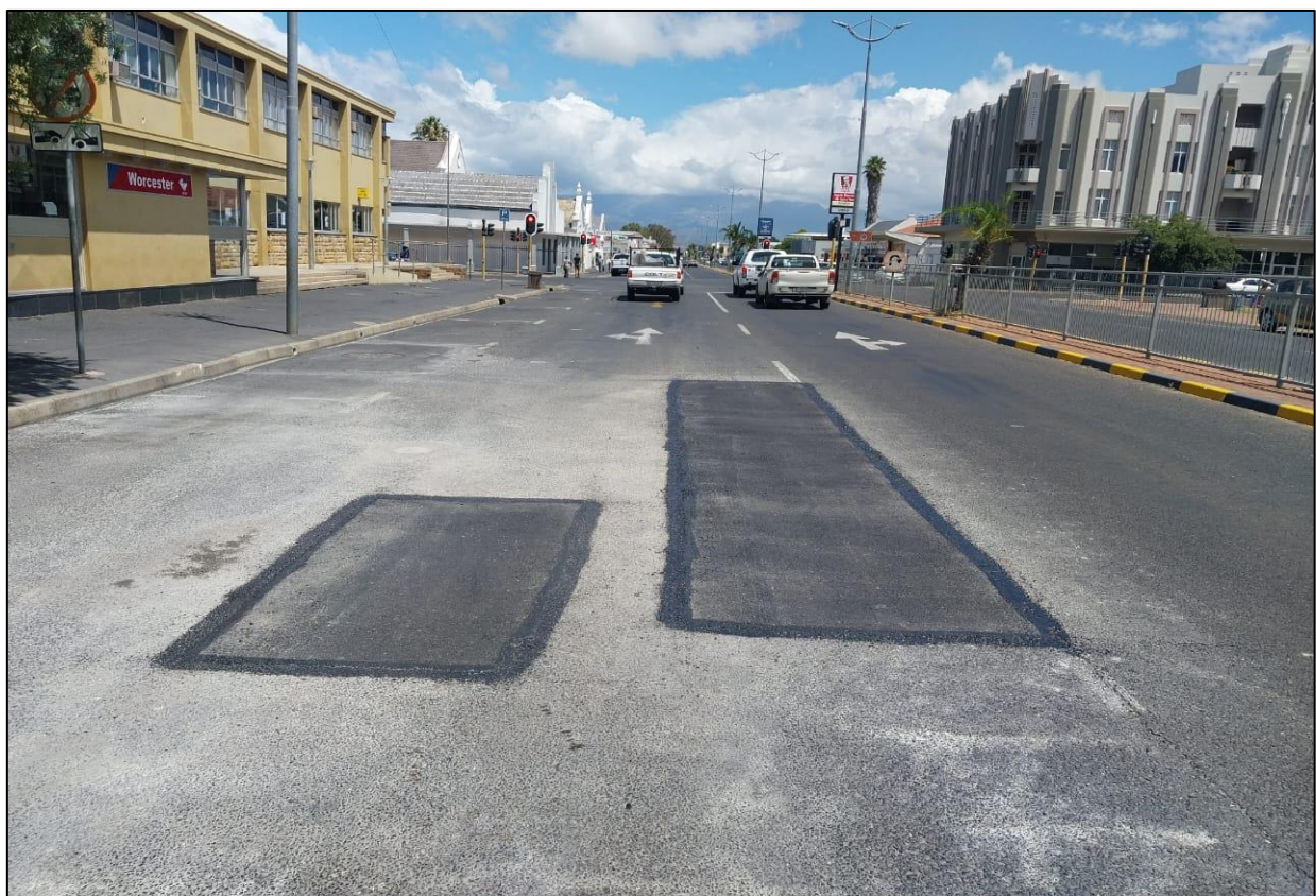
PATCH REPAIR ON HIGH STREET, BETWEEN BARING STREET AND ADDERLEY STREET (MAIN ROAD 301)
