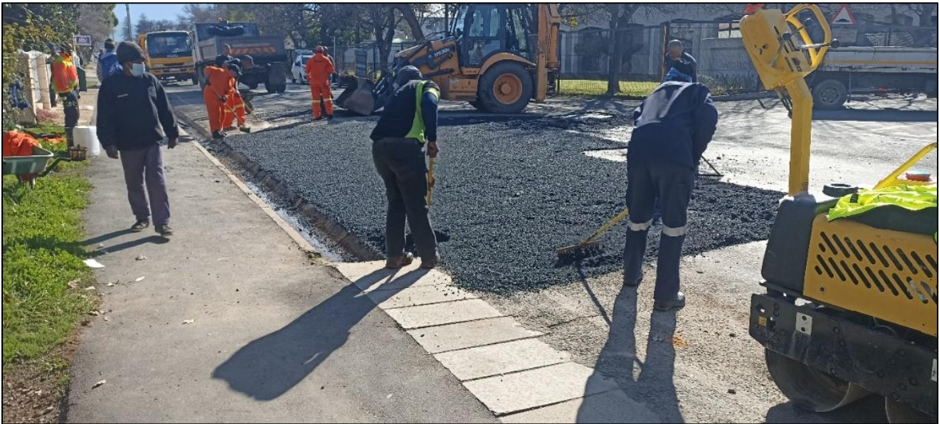
SURFACE PATCHING ON FAIRBAIRN STREET
