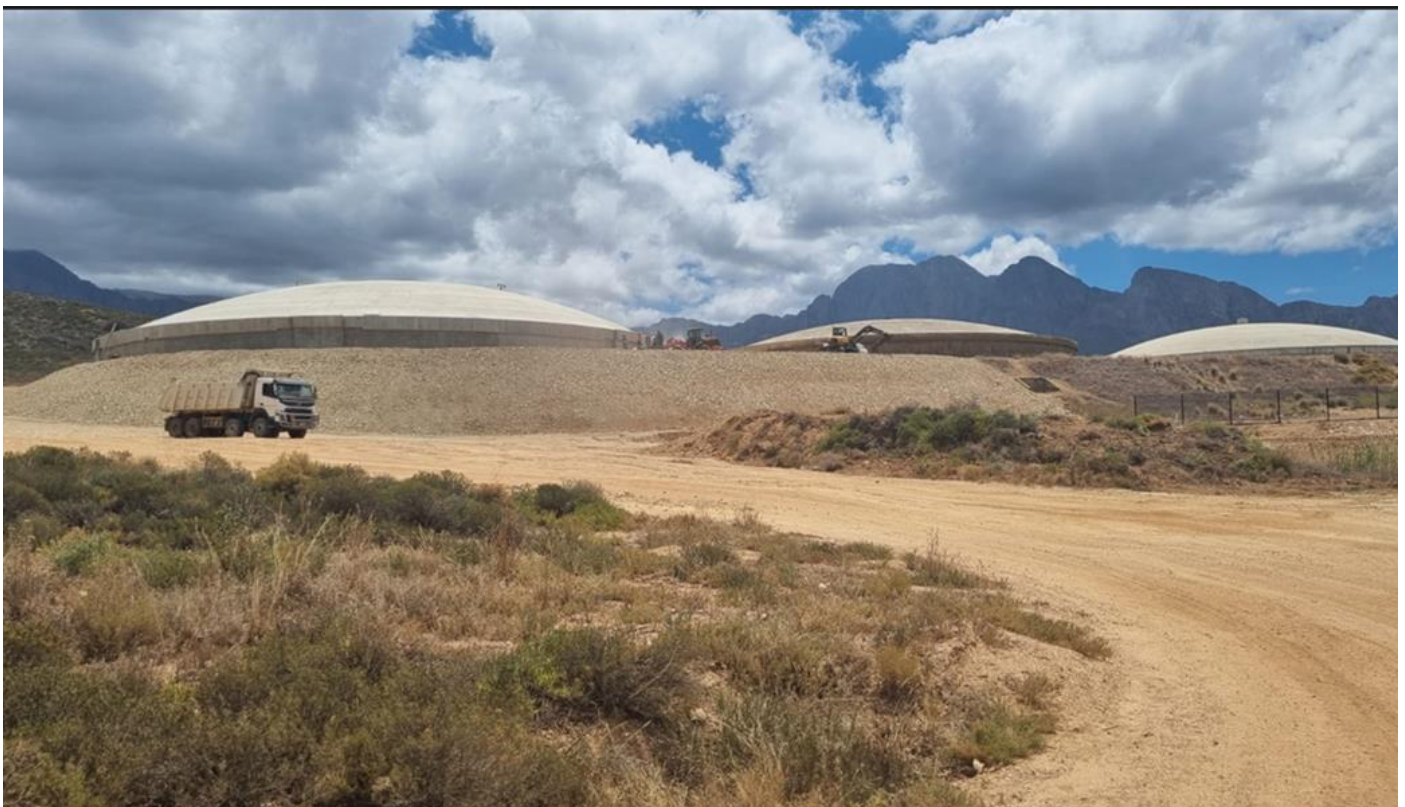
LOCALITY OF NEW 20 ML SERVICE RESERVOIR AT PRELOADS RESERVOIRS
