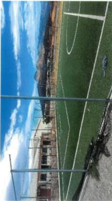
RSEP in Avian Park: derelict, vandalized, artificial turf not maintained, sections turf and fencing stolen, R750,000 wasteful expenditure.
