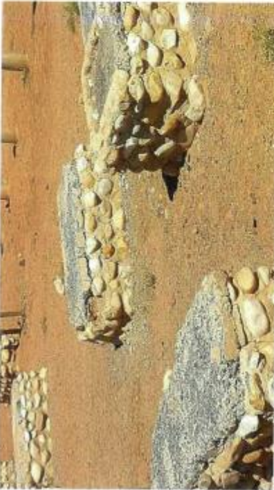
RSEP in Riverview: poorly built recreational (braai) facility, vandalised.
