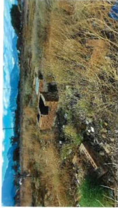
RSEP in Hexpark: recreational (braai) facility, vandalised and derelict.
