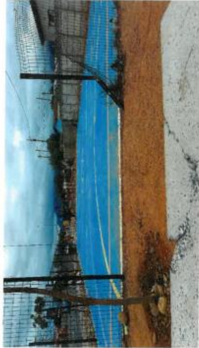
RSEP in Zwelethemba: vandalized fencing, poor quality street furniture (cracked broken concrete bench), under utilized space.
