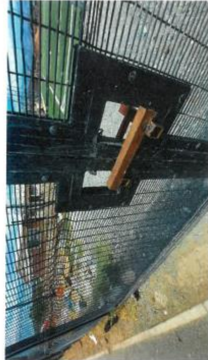
RSEP in Avian Park: gates welded shut, locked away from the community.
