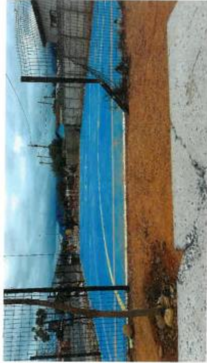
RSEP in Zwelethemba: vandalized fencing, poor quality street furniture (cracked broken concrete bench), under utilized space.
