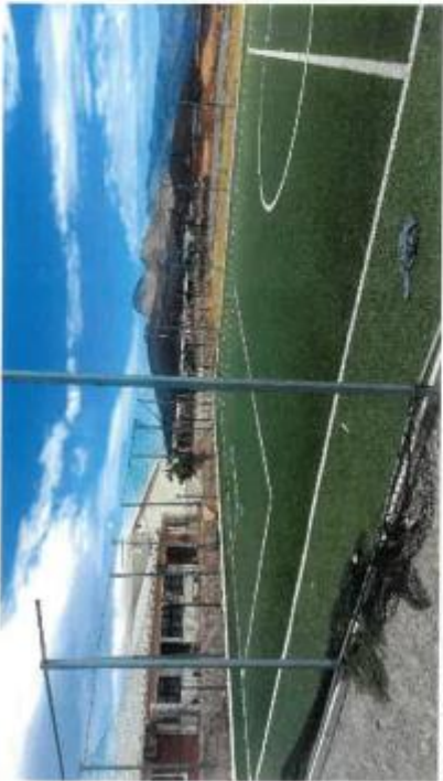
RSEP in Avian Park: derelict, vandalized, artificial turf not maintained, sections turf and fencing stolen, R750,000 wasteful expenditure.
